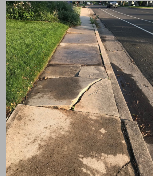
Broken or cracked sidewalks make it difficult or impossible for some users to navigate through or around.
