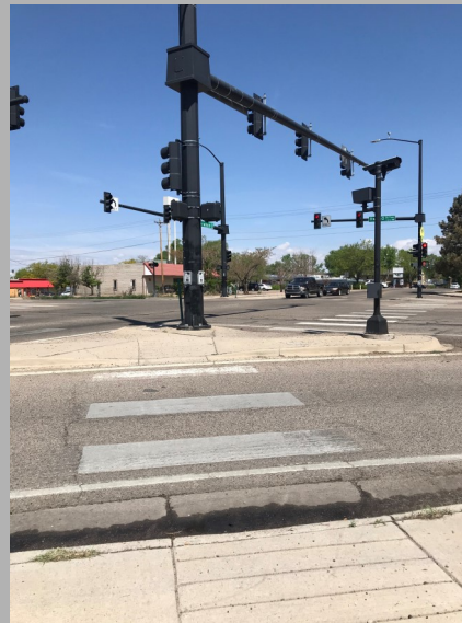
Hwy 50 By Pass and Norwood Ave. intersection needs updated ADA curb ramps
